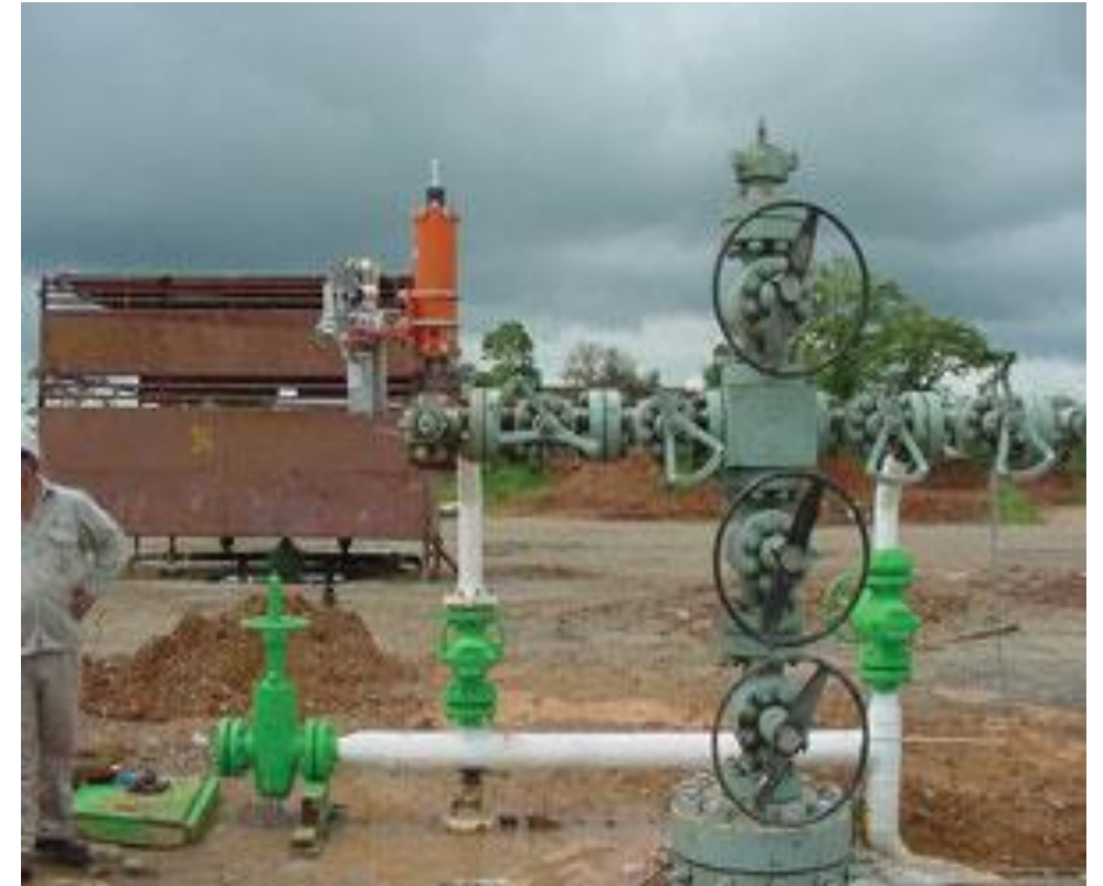
Automated Hydraulic ESD at the Choke Valve
